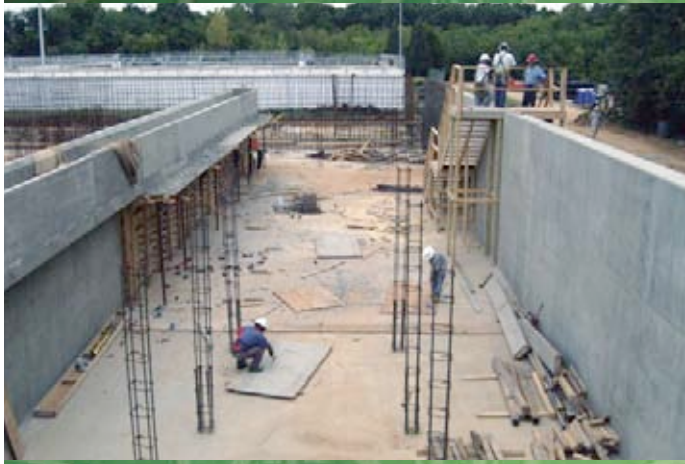
Construction began on an 8-million-gallon-a-day addition to the South Parkway Water Treatment Plant during the spring of 2008.
