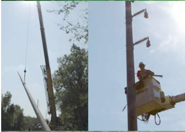
Utility poles are being installed throughout the county to facilitate growth. The crew utilizes a crane to install the pole. A line crew then installs the hardware to make the pole ready for a line when needed.
