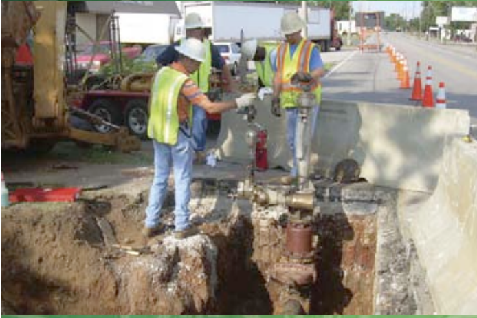
Gas Department members discuss work being done on the Brogan Branch Bridge project on Clinton Avenue with a contractor.
